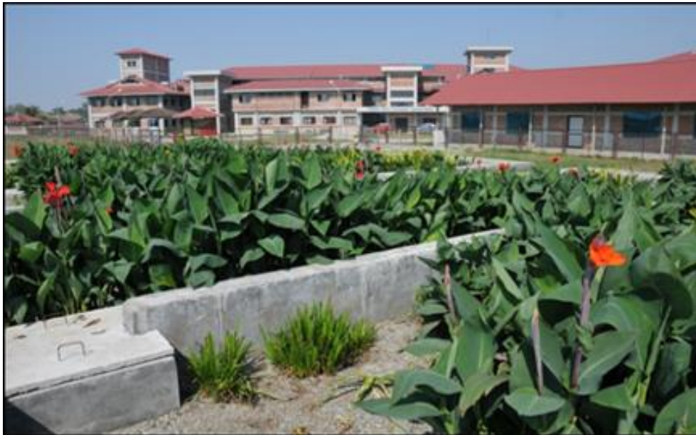
Picture 13: Decentralized Waste Water Treatment System
